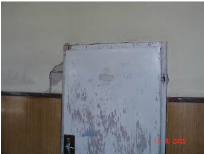
Classroom Door - Before
