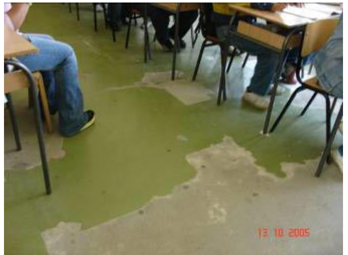
Classroom Floors – Before
