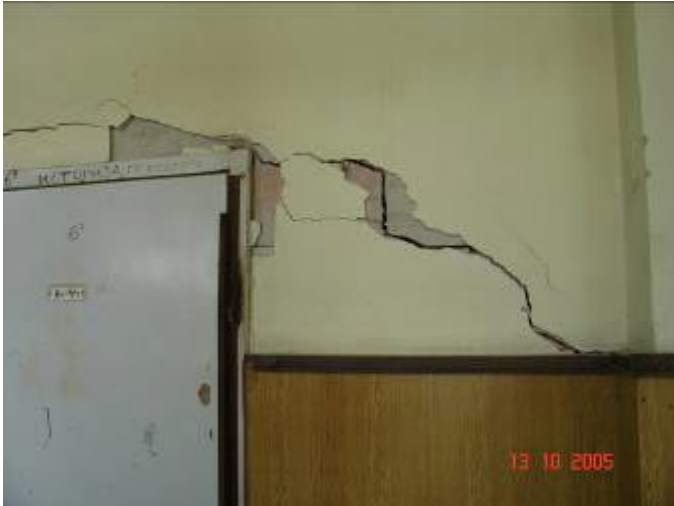
Classroom Door - Before
