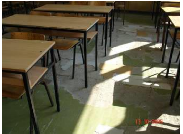
Classroom Floors – Before
