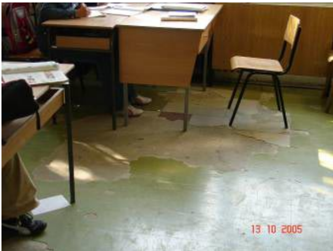
Classroom Floors – Before
