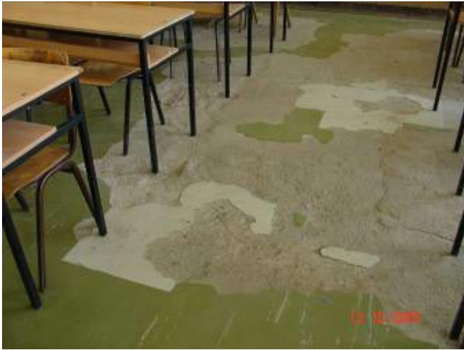
Classroom Floors – Before
