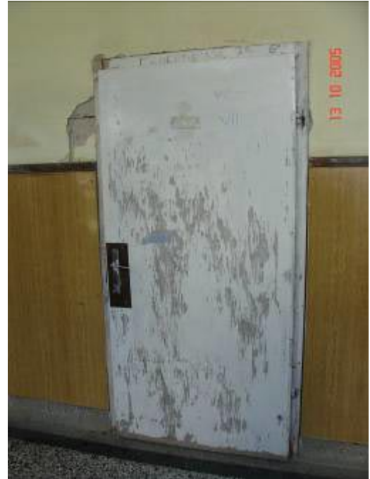
Classroom Door - Before
